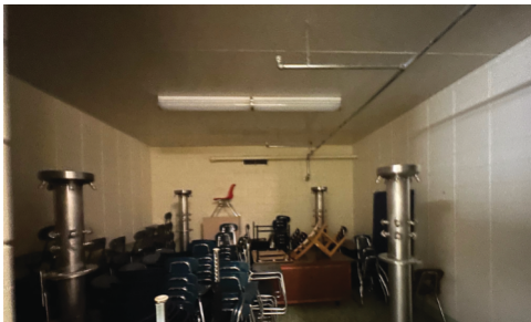
Showers used as storage
