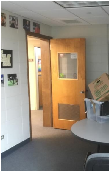
Non-ADA compliant door hardware
