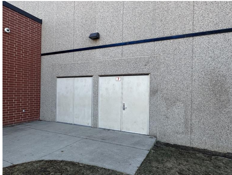
Hollow metal doors should be repainted or replaced with FRP/ALUM
