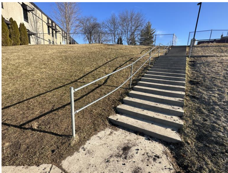
Exterior railings should be replaced
