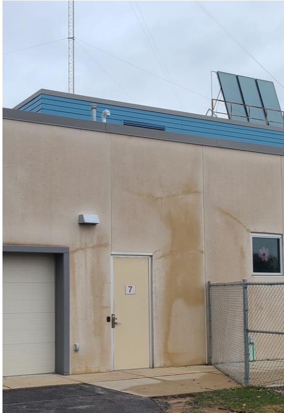
Replace card readers / maintain/seal cracks in precast
