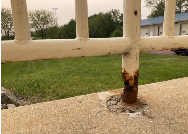
Unsafe rusted railings
